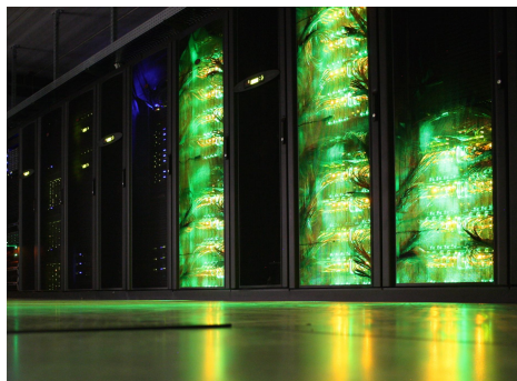
HPC-UGent Tier-2 infrastructure (2018)
